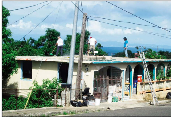
Crews work to restore a structure in Puerto Rico. The building was heavily damaged in Hurricane Maria.
